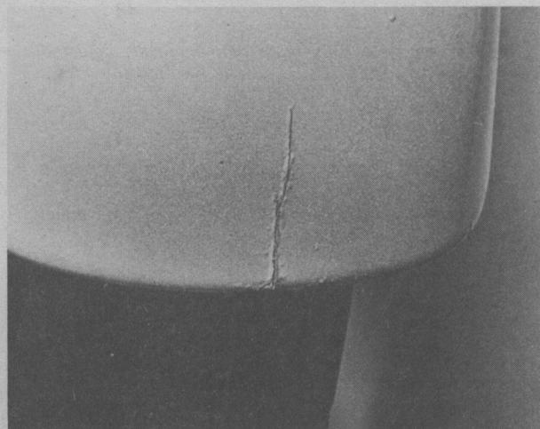
This split has been caused by vibration and will spread unless it is repaired
