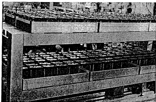
Fig. 5.64 Initial charging plant (Y. S. B.)
